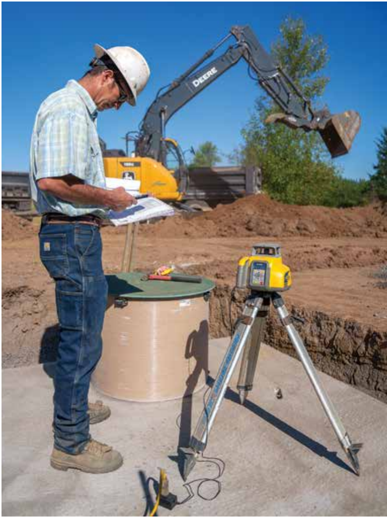
▲ Jonas reviews plans for a new system. A Spectra Precision laser level is shown to the right and a John Deere excavator works in the background.
